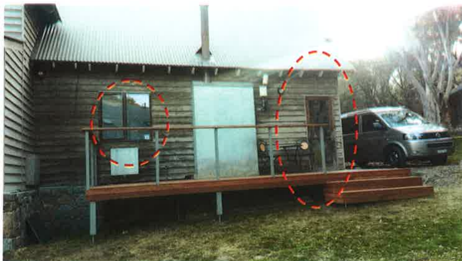
Figure 8: Photo of the eastern elevation showing the existing door to the deck and window to be replaced.
